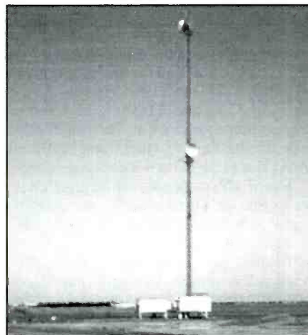
Microwave relay tower on Tap line road. Thanks to "The Sarge."
