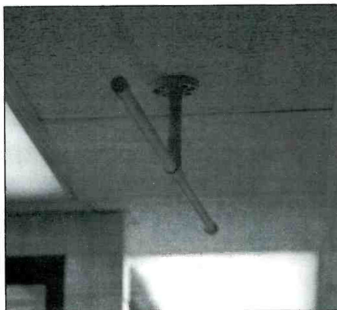
This antenna was spotted installed at a fast-food restaurant. Turned out to be used with the establishment's low-power 35.02/154.60 MHz communications system.
